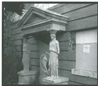
These caryatids at the 1914 Nueces County Courthouse have been neglected for more than 20 years. Because of a deed restriction held by the THC, the building is still standing and has received Round II funding.
